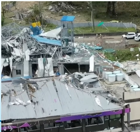
Photo: Drone shot showing damage caused by the CCCL explosion
